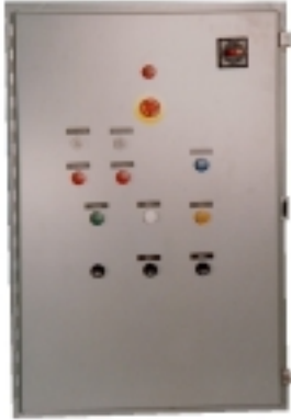
PLC Control automatic or manual operation
